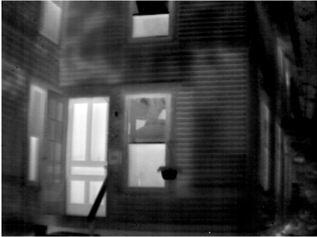
The quality of the images produced by modern IR systems is remarkable. Missing and poorly installed insulation is easily seen.
