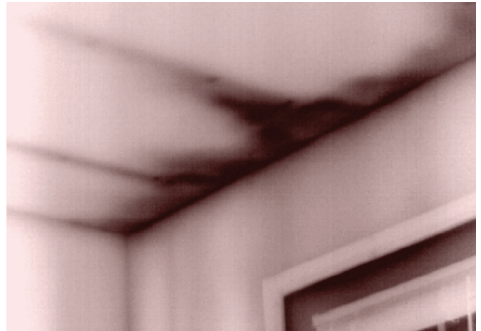
Air wash along the edges of batt insulation produces a unique cold signature on the ceiling of this wood-frame commercial building.
