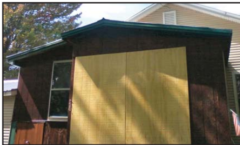
Image 8. Was there missing insulation here?
