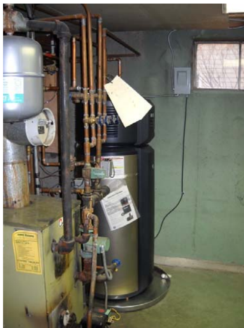
Figure 4. Waste heat from this boiler kept the basement mechanical room very warm all winter, and the HPWH was able to operate quite efficiently.
