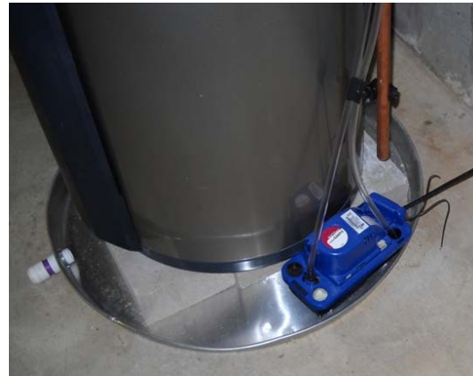
Figure 6. Water heater installed on blocks within drain pan.
