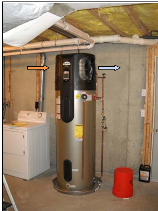
Figure 3. Heat pump water heater with appropriate clearance for air movement.
