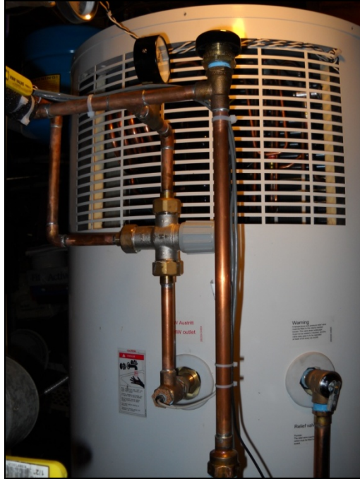
Figure 8. Heat pump water heater with a tempering valve.
