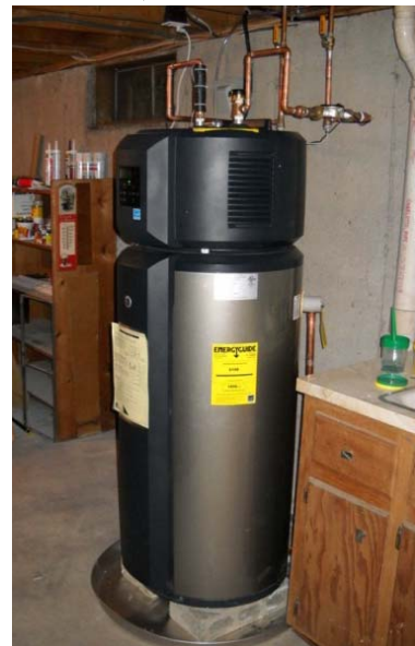
Figure 1. An integrated HPWH installed in a basement.
