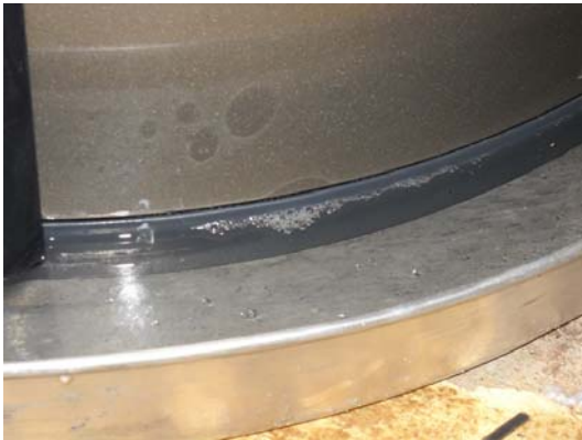
Figure 5. While this heater was installed in a drain pan, it was not on blocks. When a condensate drain problem occurred, the water heater was sitting in an inch of water.
