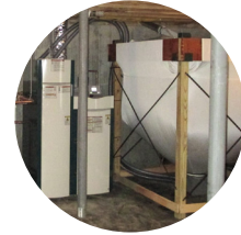
Central wood pellet furnaces and boilers
